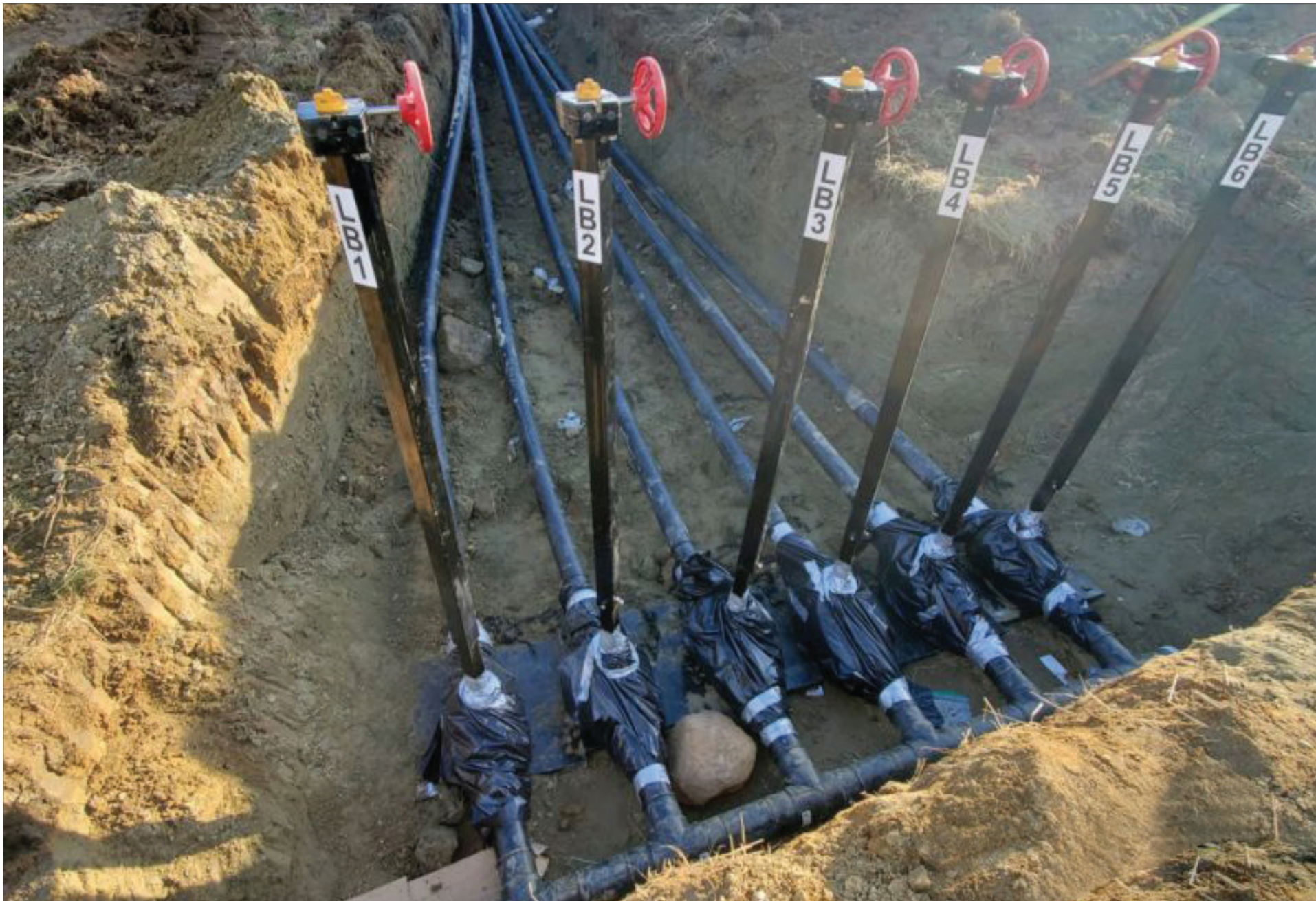
Asahi/America's Type-57P butterfly valves installed in a landfill application. Optional stem extensions were added to the butterfly valves by Asahi/America for this hard-to-reach application.
