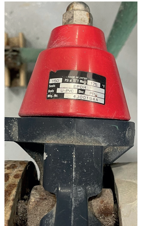
Asahi/America's Type-75 PVC butterfly valve (installed in an aquarium application for over 25 years. (The manufacturer number on the lever of the butterfly designates the year in which the valve was made. Here it shows 4J00194A, meaning this valve was manufactured in 1994.)
