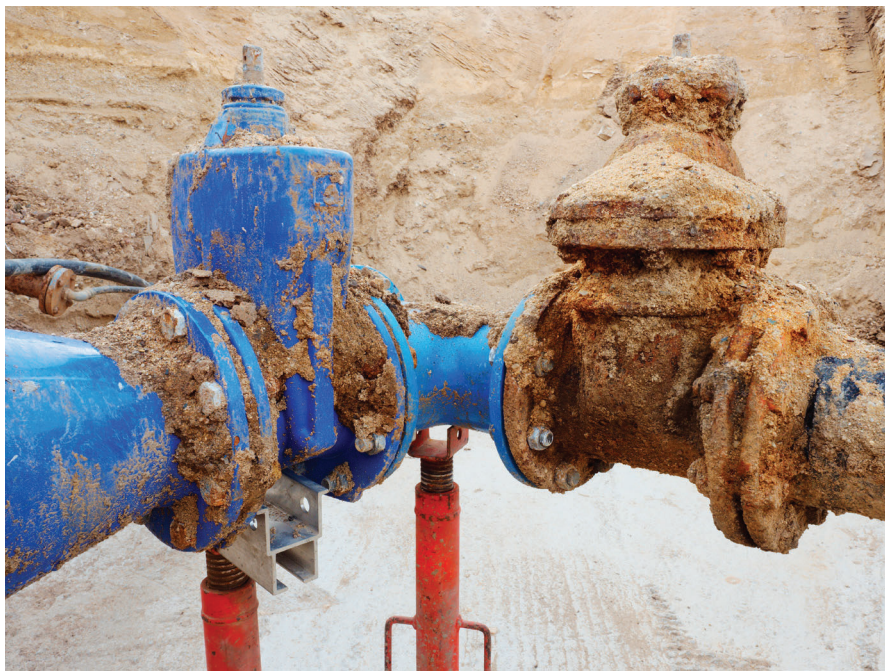
Corrosion attacking a coated metal valve.
