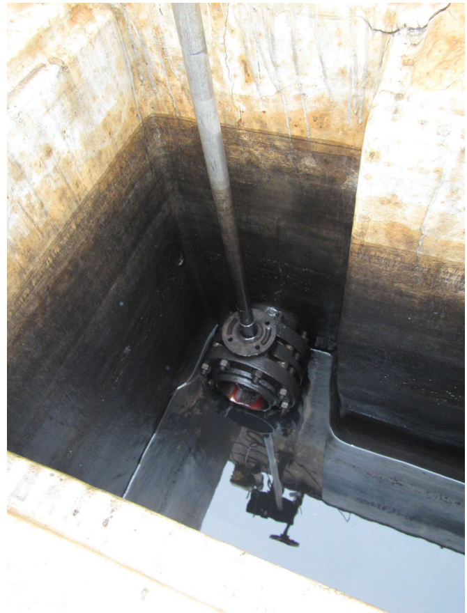
Extension stem on an Asahi/America Plasgear™ operated Type-57P butterfly valve that replaced a corroded metal stem and valve installed in a drain application.
